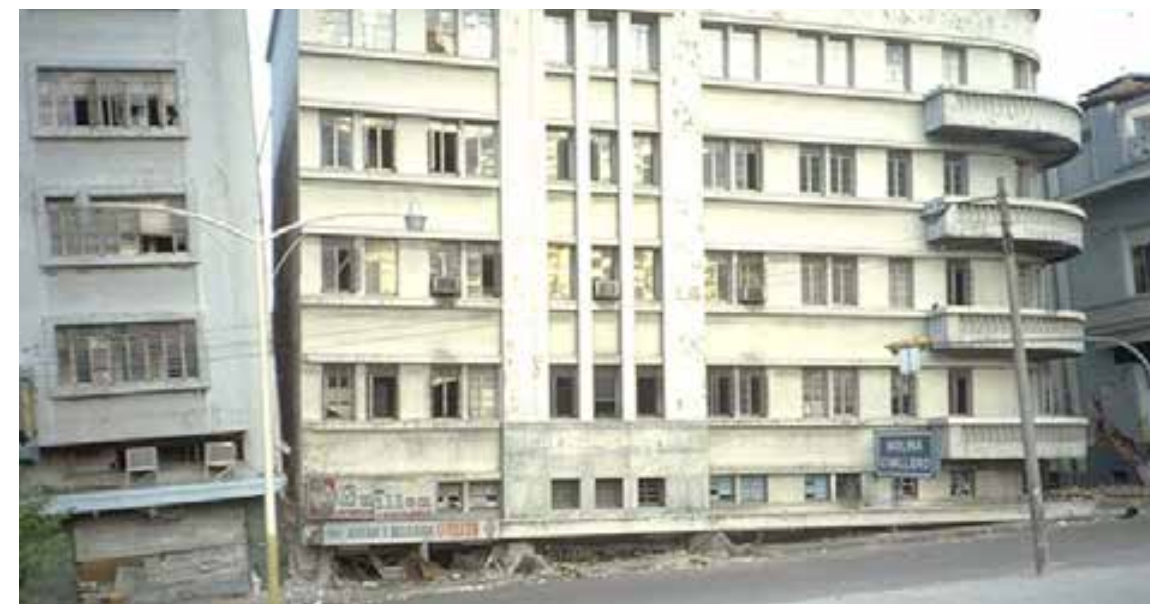
Figura 135. Daños observados durante el sismo de 1986, M5.7 – San Salvador 61 Fuente: Olson, Robert A. Collection. Earthquake Engineering Online Archive, National Information Service for Earthquake Engineering, EERC, University of California, Berkeley
